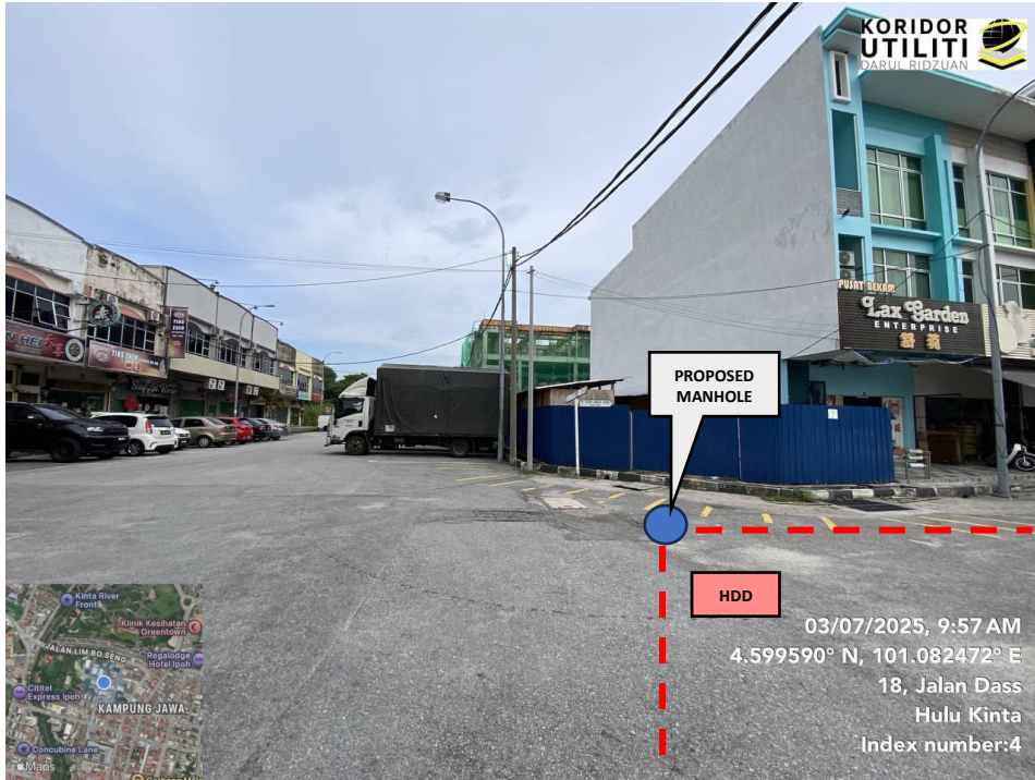
JAJARAN KERJA HDD DI JALAN HORLEY (Tapping from new manhole 1 to new manhole 2)
