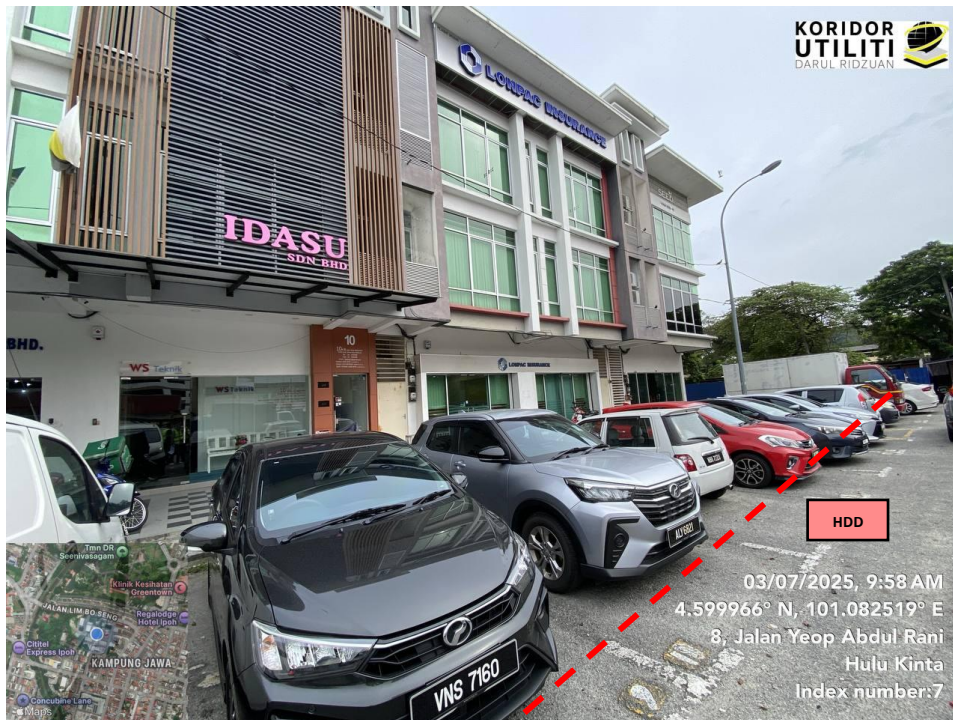
JAJARAN KERJA HDD DI JALAN YEOP ABDUL RANI (Tapping from new manhole 2 to existing manhole)
